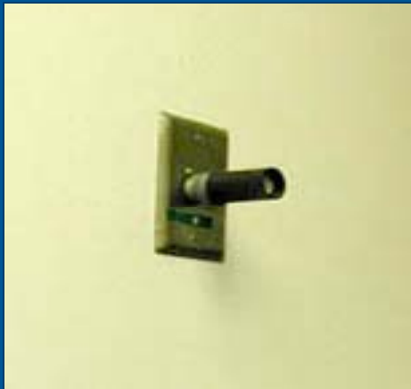
EtO Room Monitor
